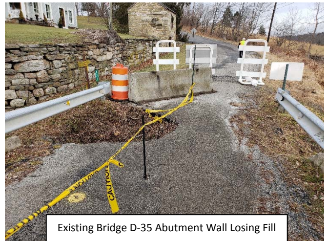
Existing Bridge D-35 Headwall Failure
