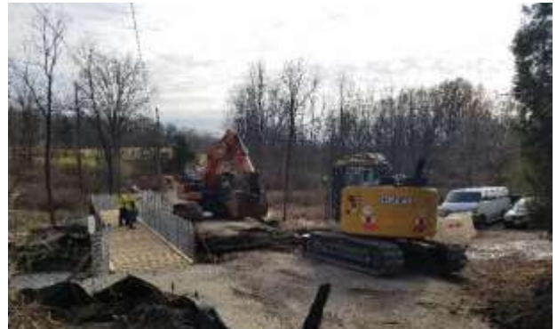
Bridge D-21: View of Existing Bridge Demolition and Pedestrian Bridge Looking East
