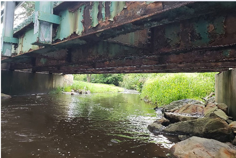
Bridge X-54: Typical Steel Deterioration
