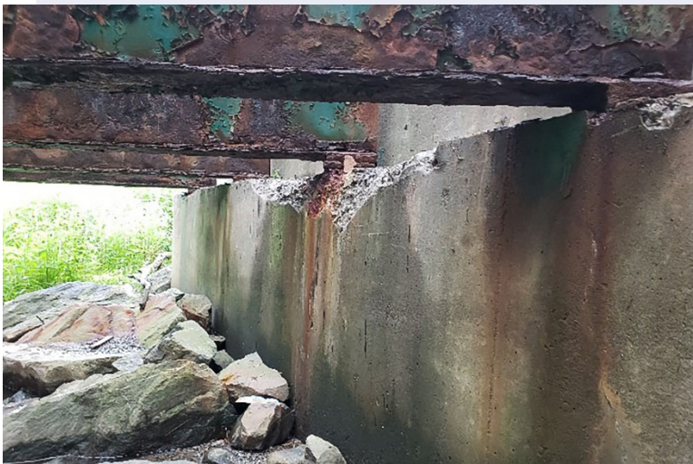
Bridge X-54: Typical Concrete Spalling and Steel Grider Deterioration at Bridge Seats
