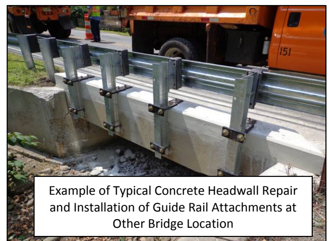
Bridge H-19: Downstream Headwall. Note Need for Headwall Repairs and Guide Rail Attachments
