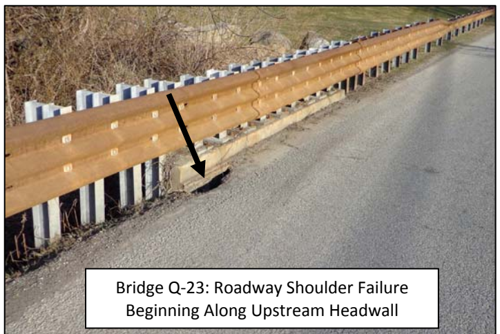
Bridge Q-23: Slope Erosion Along Upstream Headwall and Roadway Shoulder
